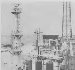
Sour Water Stripper.
